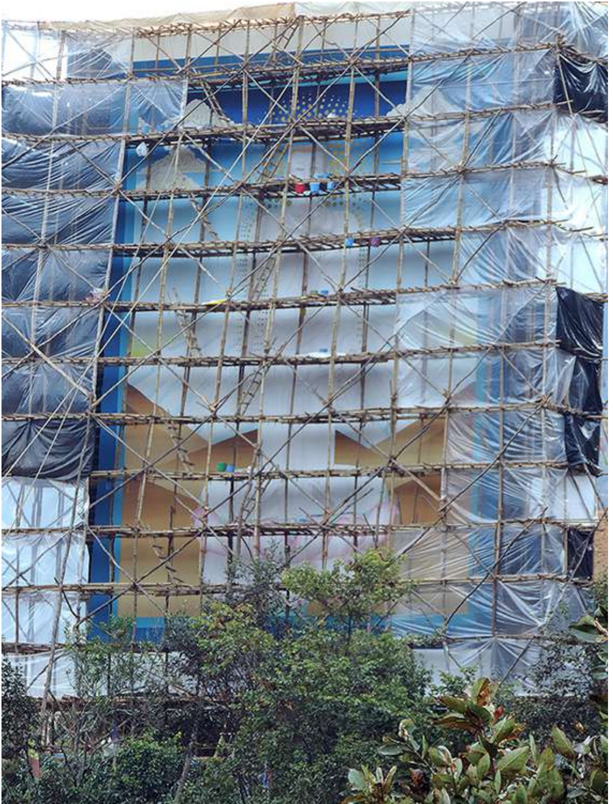
The 85-foot Mahā Maitri Mārgaguru thangka was affixed to this 100-foot bamboo scaffolding erected on a hillock at the Badegaun Maitri Precinct, where painters climbed up each day to work on their respective areas. (Sindhupalchowk 2015.)
